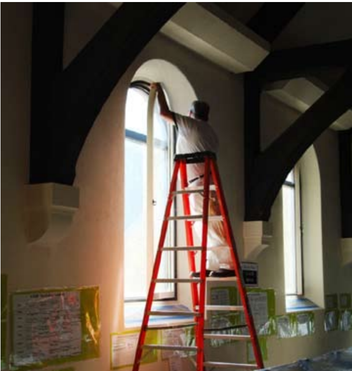
All of the windows in the Sanctuary, Ames Chapel, and Parish Hall are being restored.
