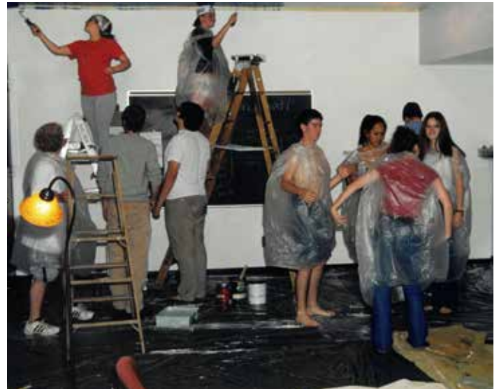
Youth work project, painting classrooms, ca 2002. Very creative use of trash bags as protective covering!
