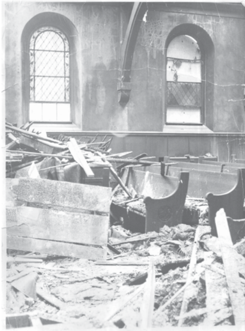
Views of fire damage and rebuilding efforts, 1963-1964. Unity Church Photographs and Negatives Collection. Minnesota Historical Society, Saint Paul, MN.
